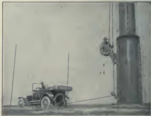
The other end of the cable is fastened to a moving automobile which is hoisting the jack three hundred feet to the top of the mast
